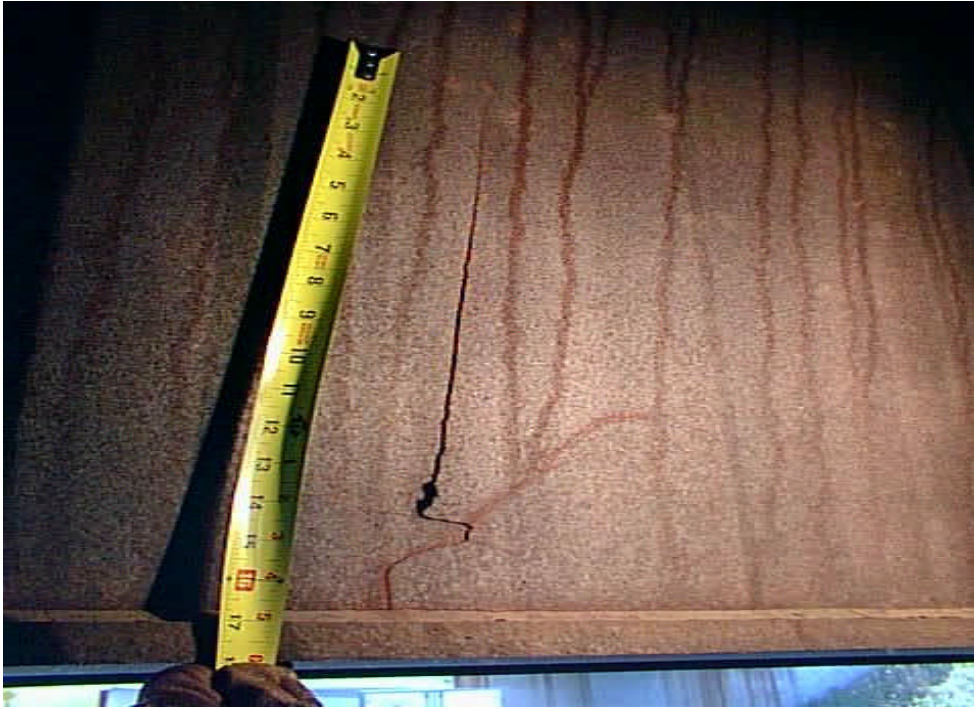
Photo: Cracks at one box girder web. Web to bottom flange connection was also cracked completely through
