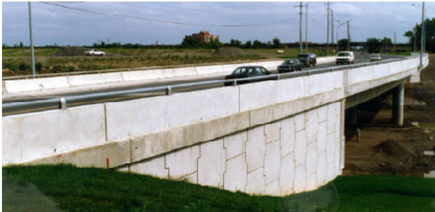
Islington Ave. bridge over Highway 407 open to traffic. Note the precast wingwall and abutment face details.
