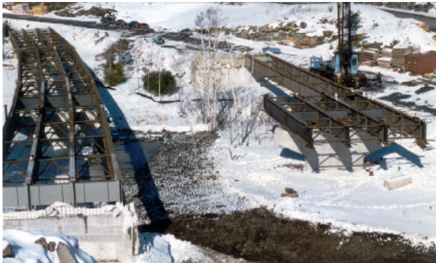
SBL structural steel erection completed and NBL pier segments in place with erection of north span girders in progress.
