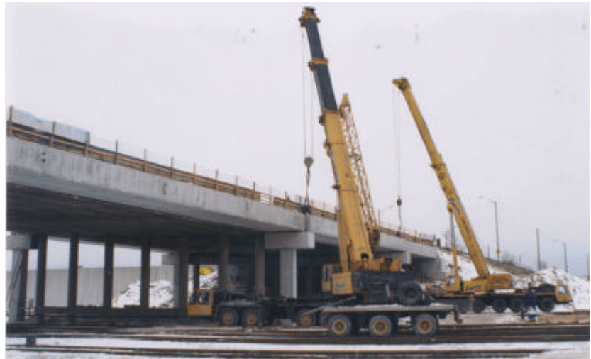
Erection of prestressed box girders for the Markham Road bridge widening. This is a five span structure, longest span 33.5 metres.
