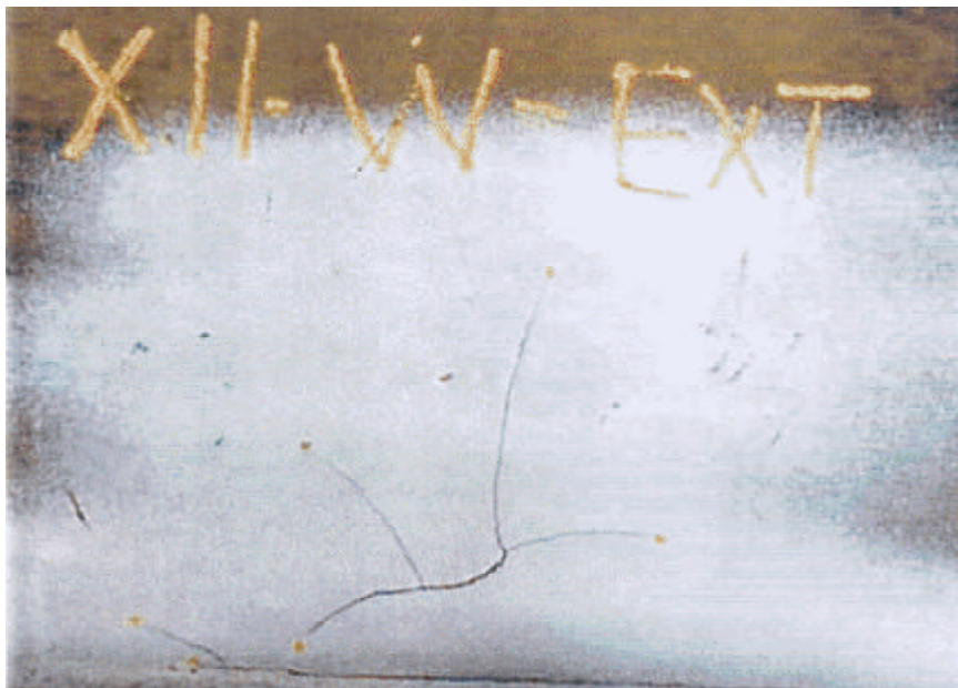
Typical distortion induced cracking at box girder web viewed from outside.
