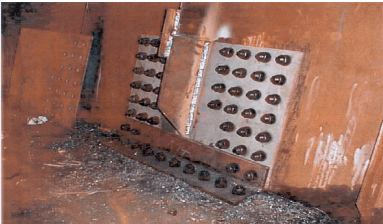
Typical web repair plate assembly inside box-girder, note also stiffener restoration and bottom flange connection.
